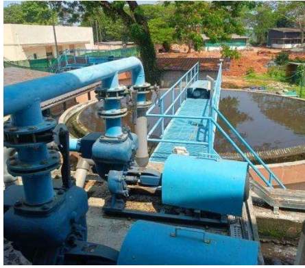
500 KLD STP at Kozhikode medical College
