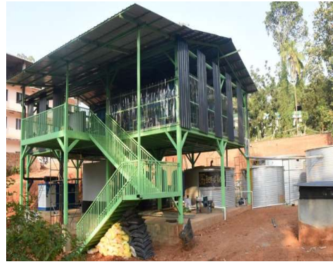
1 MLD STP at Kozhikode medical College
