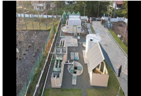
1 MLD CSTP at Padanappalam, Kannur
